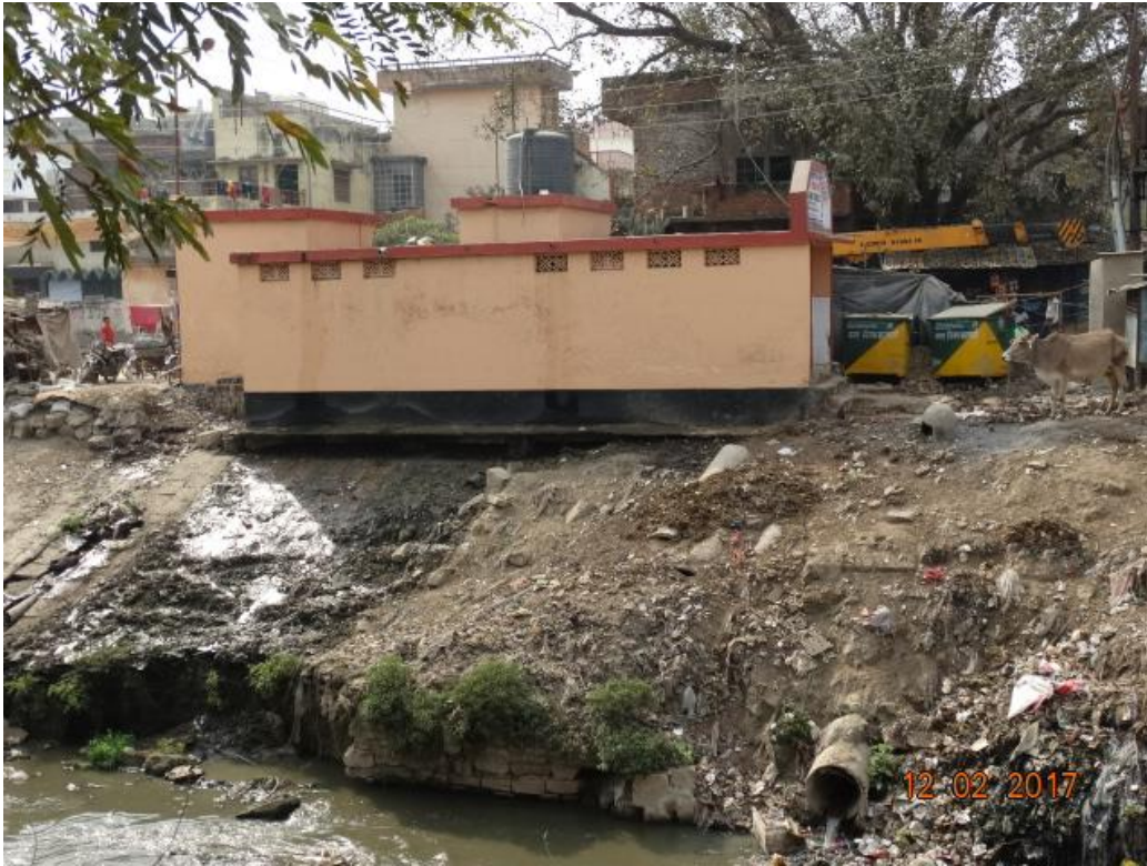
Image 10 : Sewage Leaking From Sulabh Shauchalaya Eroding Own Foundations [Note: Another Inflow At Bottom of Image]
