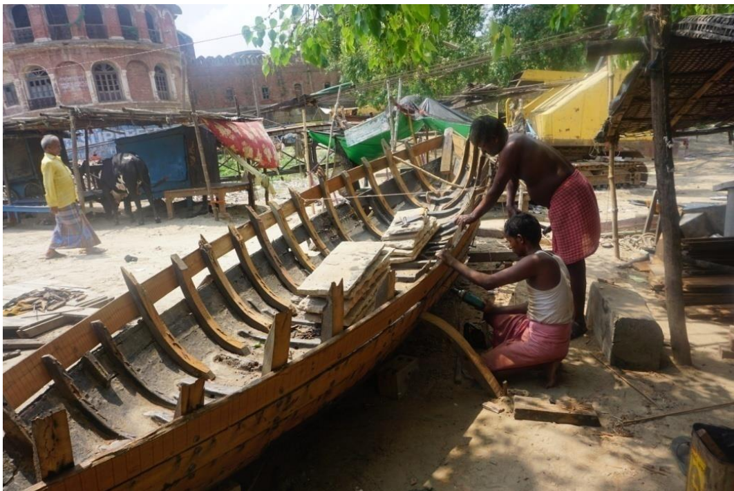
Image 71 : Construction Of A Small Sized Boat By Mallah Community Near Ramnagar Fort
