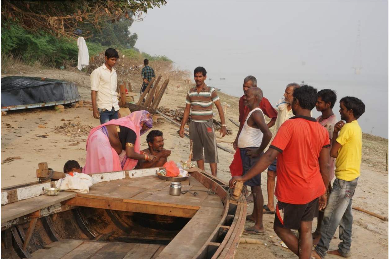
Image 72 : The Owner Of A Newly Constructed Boat Performing Puja Before Launching His Boat In The River
